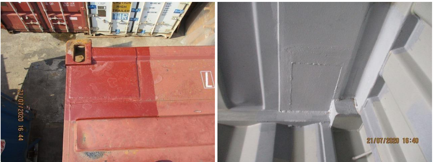
Proper replacement of the corner protection plate after installation of insert on the extension plate.
