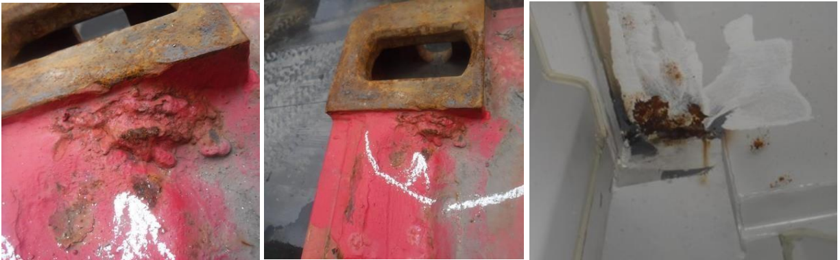
Non-conforming repair. The damaged area filled with weld without restoring original profile of the rear Header and corner protection plate.
