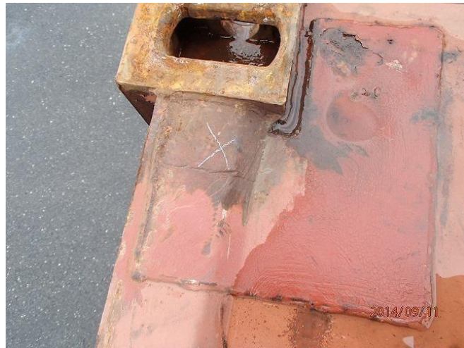
Acceptable insert on corner protection plate. Any damage to the front header must have been repaired prior to insert installation. Repair shall not protrude above the upper face of the corner fitting.
