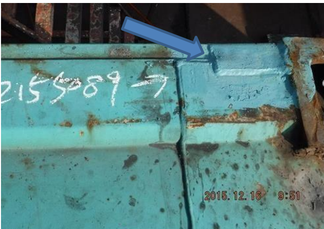
Non-conforming patch to the corner protection plate, overlaps the front header.
